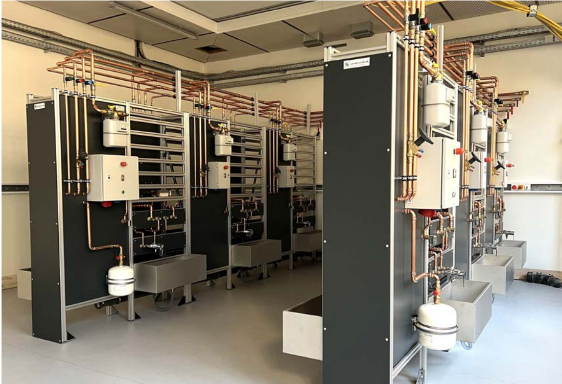
Gas training laboratory: workstations for supplying heat generators (gas condensing units, heat pumps)
