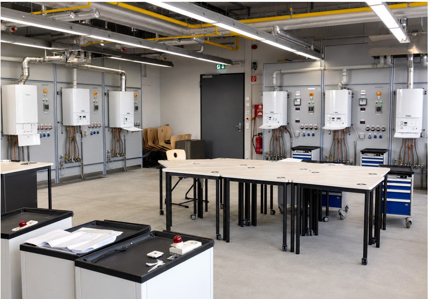
Technical laboratory for gas appliance training
