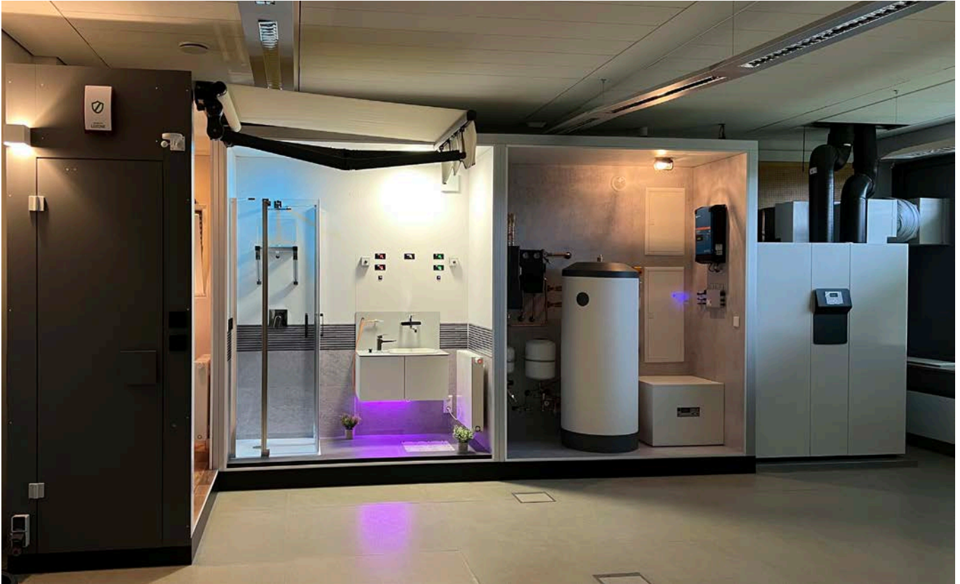
Training wall "Digital Building Systems" featuring an integrated valve testing station in the bathroom; the building automation is realized using Loxone components.
